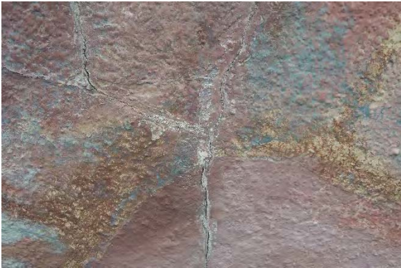
Example of Weathering and Damage
