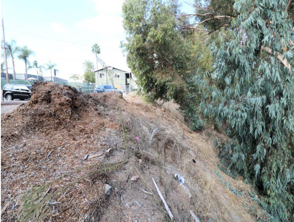
Partial view of the steep slope on the northern portion of the site.
